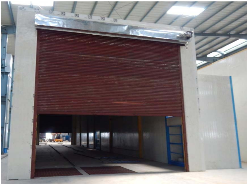
Painting Booths – (5 Nos.)
