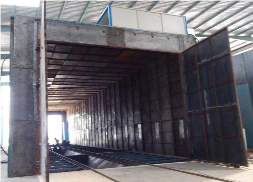
Blasting Booths (3 Nos.)
